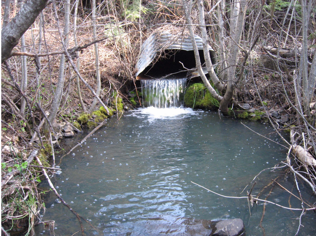
Figure 11.11. Culvert outlet drop at the Stahl Canyon road crossing within the Umatilla National Forest (Wheeler County), Buckhorn Creek subwatershed, Oregon.
