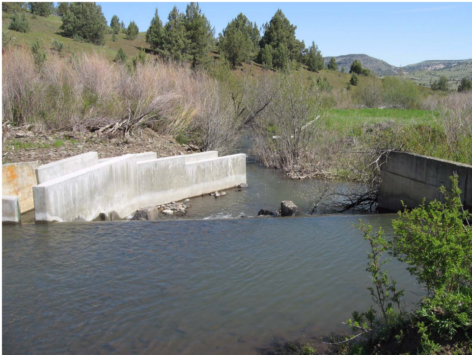
Figure 11.9. Diversion dam on mainstem Buckhorn Creek with recently installed fish ladder, Buckhorn Creek subwatershed, Oregon.
