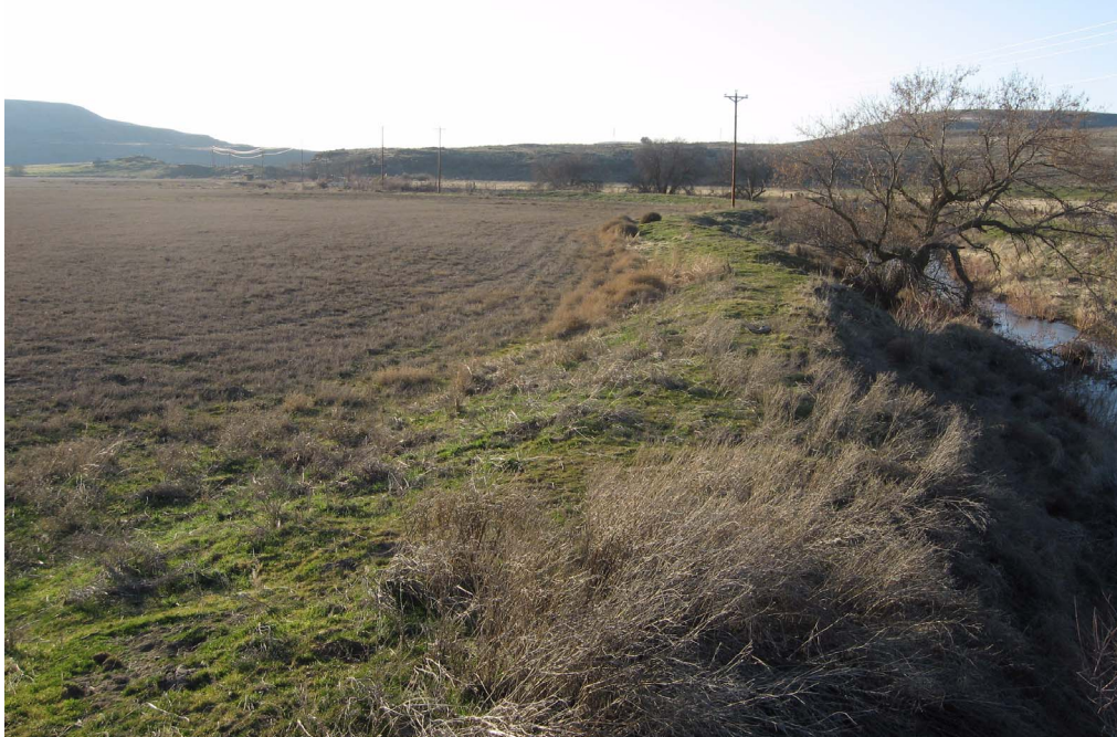
Figure 9.2 Dike along a channelized portion of lower Rock Creek in the Rock Creek and Lonerock Creek watershed, Oregon.
