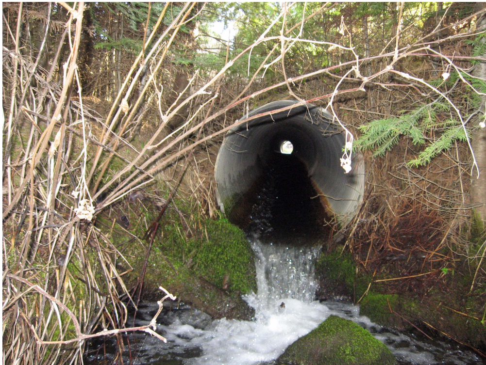
Figure 11.12. Culvert outlet drop at the Wineland Creek road crossing within the Umatilla National Forest (Wheeler County), Buckhorn Creek subwatershed, Oregon.
